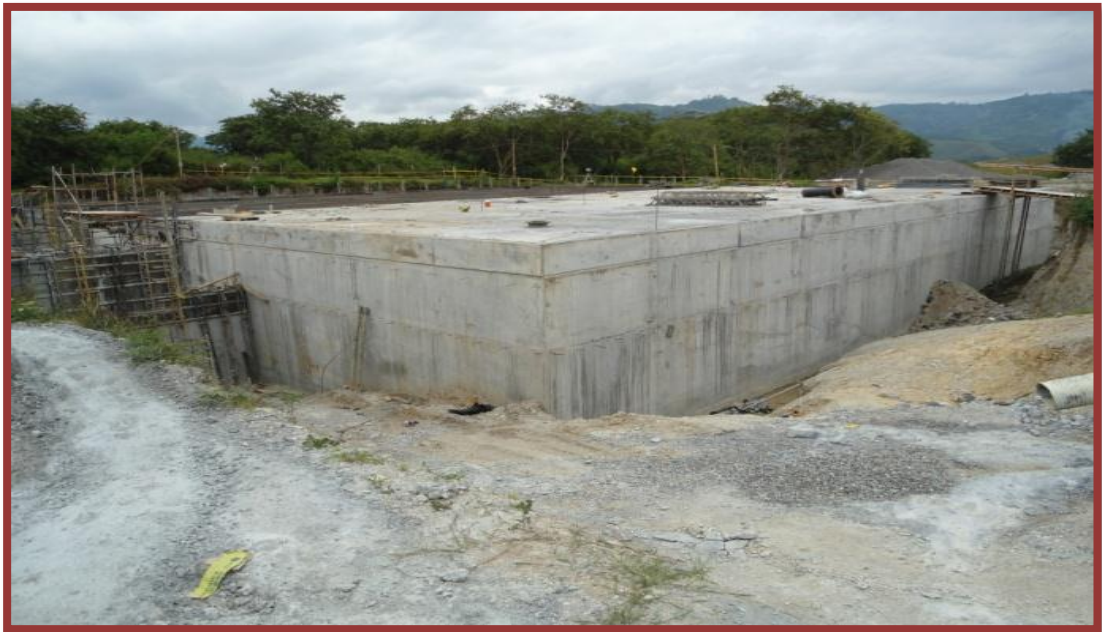
Vista general Tanque No.1 PITALITO PTAP
